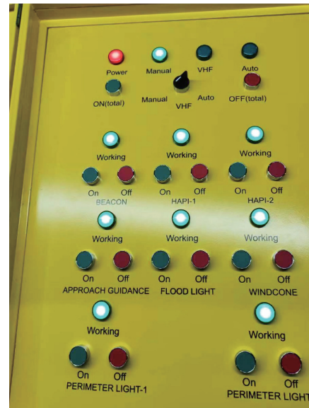
Example of control panel(Internal panel)
